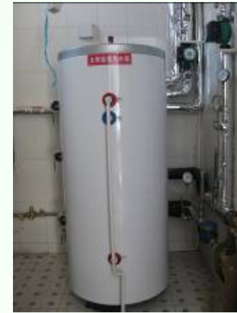
Heat storage tank
