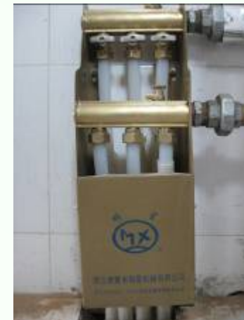
Water segregator and collector
