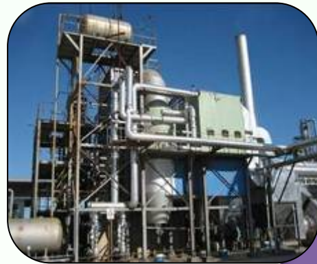
North Town heating
