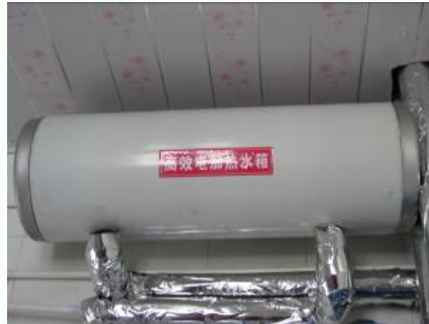
Electrical heating water tank
