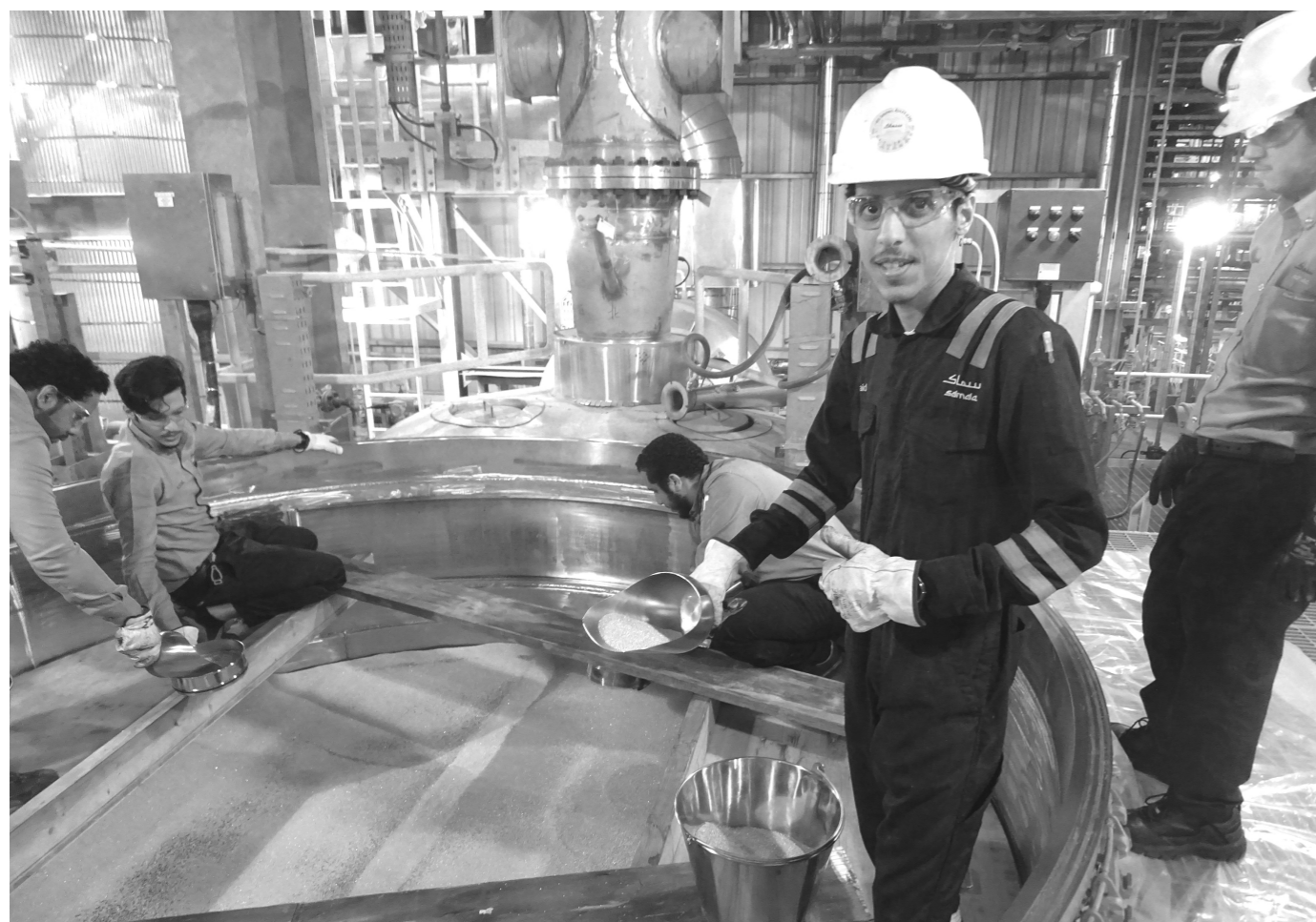
Catalyst filling in a new process unit. How the reactor is filled is crucial for the process performance. Filling procedures are based on process and catalyst knowledge combined with decades of operational experience.
