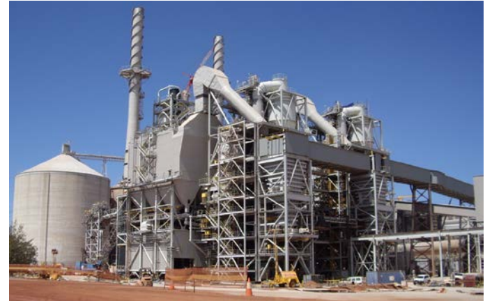
Rio Tinto Alcan Gove 3 CFB calciners.
