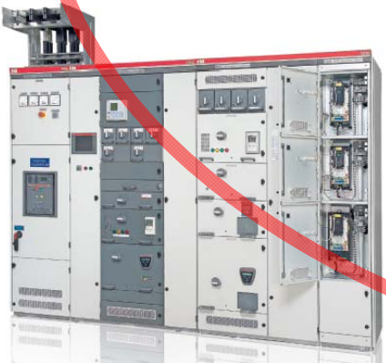
Low voltage switchgear for microgrid modelling
