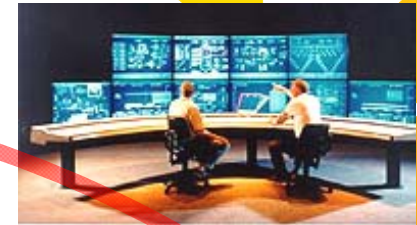
Supervisory Control and Data Acquisition system for monitoring, controlling and data collection (also from remote sites)
