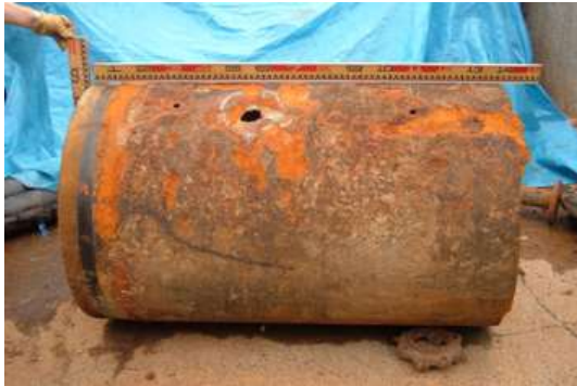
deteriorated pipes dug up in Yokohama
