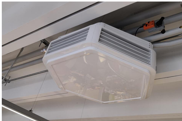
Figure 2: Heating and AC terminal unit in the shopping area
