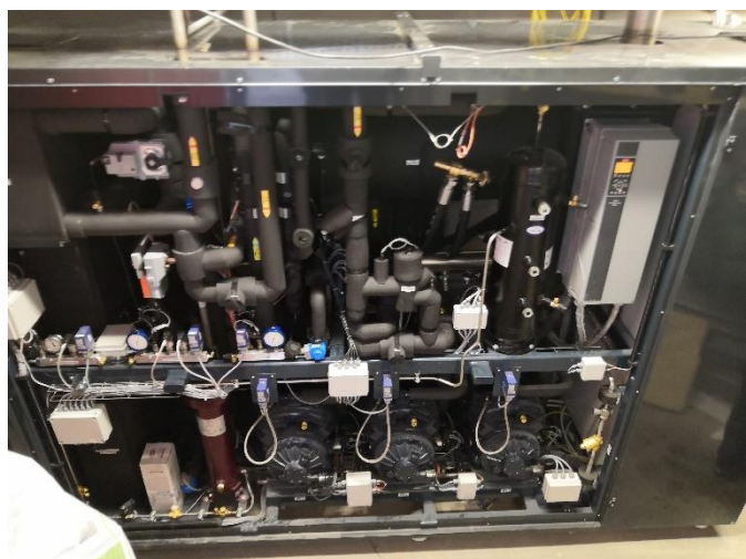
Figure 1b: Val Gardena unit (SITE II) as installed in the field
