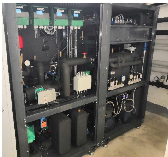
Figure 1a: Garda Lake unit (SITE I) as installed in the field
