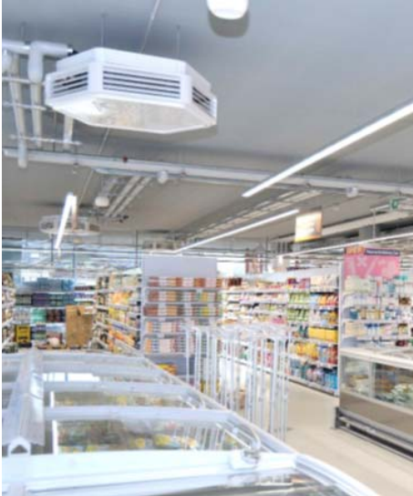
Figure 8: Direct heating and cooling fan coil unit inside a Supermarket (Giroto 2016).
