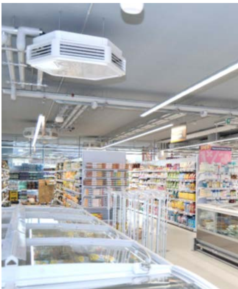
Figure 6: Direct heating and cooling fan coil unit inside a Supermarket (Giroto 2016).
