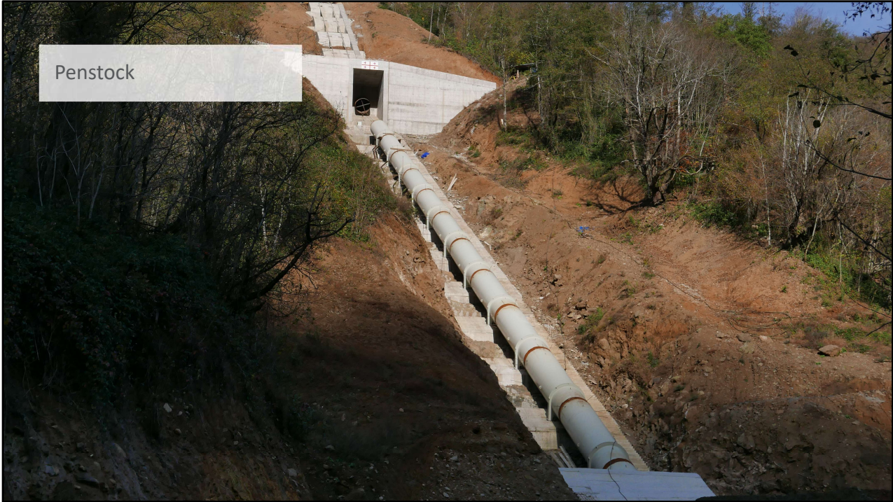
From the tunnel we have a superficial steel penstock of approximately 500 m in length and...*
