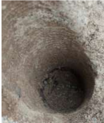
Figure 7. Intact borehole at the bottom of the failure crater after anchor B1.5m.
