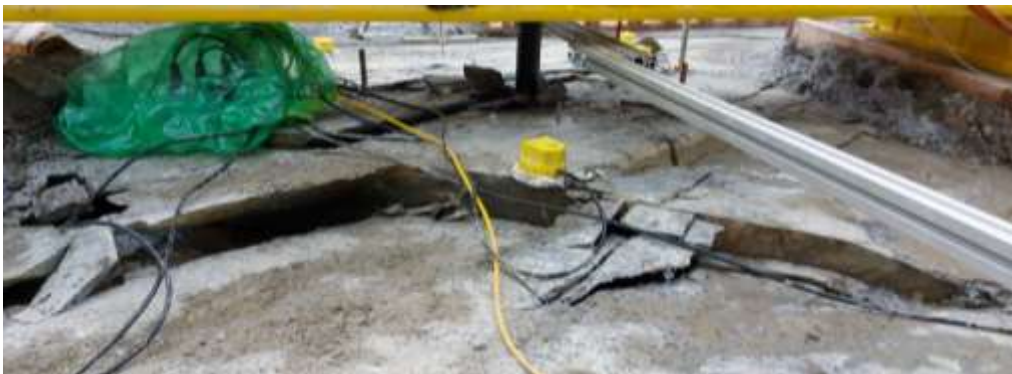
Figure 9. Surface cracking around anchor B1.5m after the test finished.
