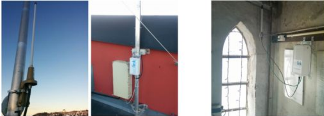
Figure 9 Deployment of LoRaWAN antenna gateway outdoors on the roof of the Student Society building in Trondheim (left) and elevated indoors in a clock tower in Vejle (right)
