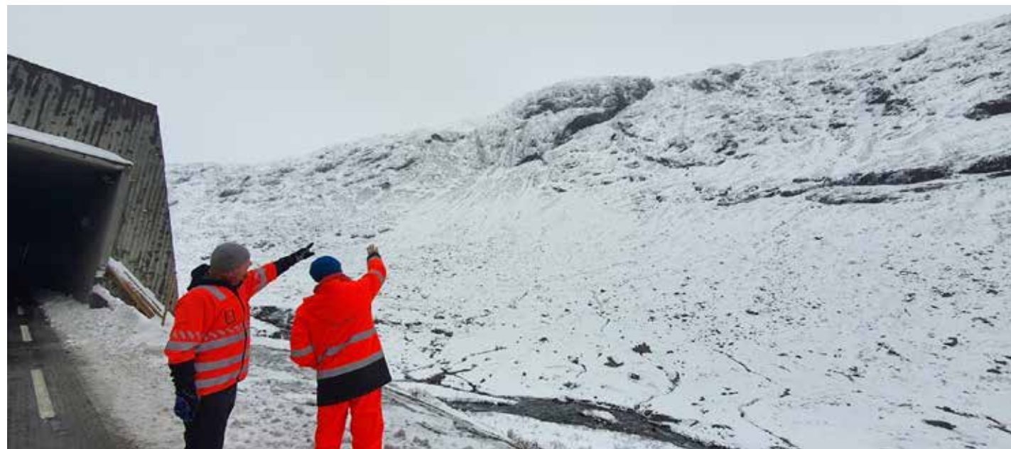
Figure 14. Experts at the tunnel entrance, inspecting the slopes with potential avalanche paths.
