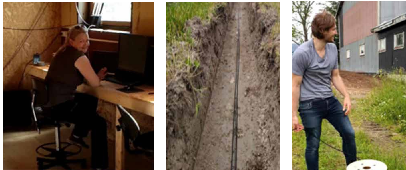
Figure 2. Preparation of DAS data acquisition with interrogator in the barn, installation and trenching of fiberoptic cables.
