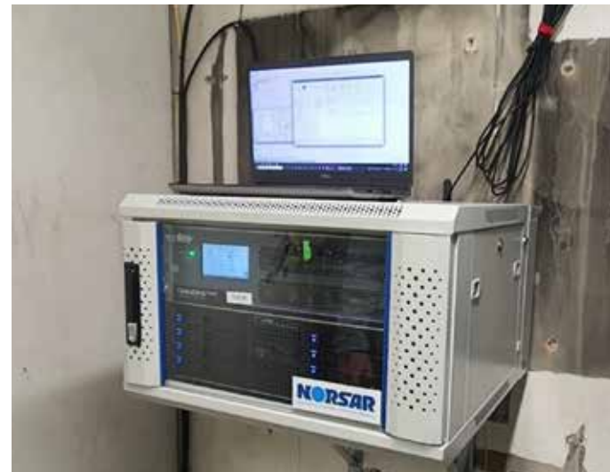
Figure 15. DAS interrogator unit installed in the tunnel at site K6.
