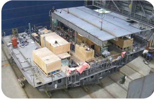
Machinery and generators (covered in wood boxes) are already outfitting on the steel or structural block.
