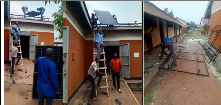
The process involves hiring local welders to weld the frames and install solar panels
