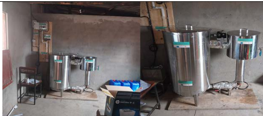
The installed system in the kitchen at Pagirinya SS.
