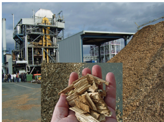
The Güssing 10 MW biomass gasification reactor, a hub for biofuel research in Europe
